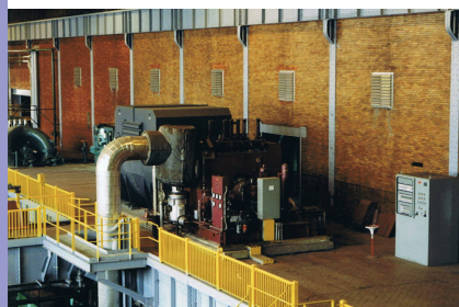
22 MW Synchronous Unit
