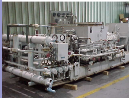
1 MW Synchronous Unit
