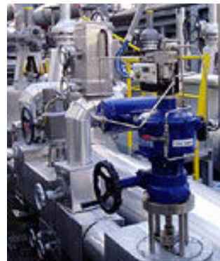
STEAM PRESSURE REDUCING STATION
